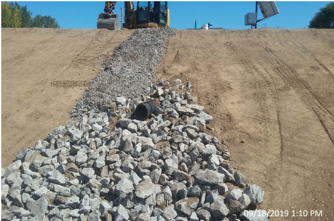
Photo 65- Settling Pond Inlet Pipe Stone Rip Rap and Access Path
