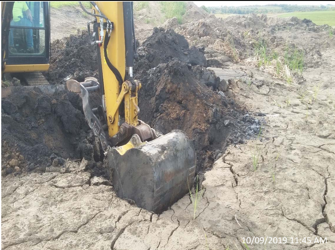
Photo 66- Sediment Mixing with Underlying Fly Ash in the Confined Disposal Area
