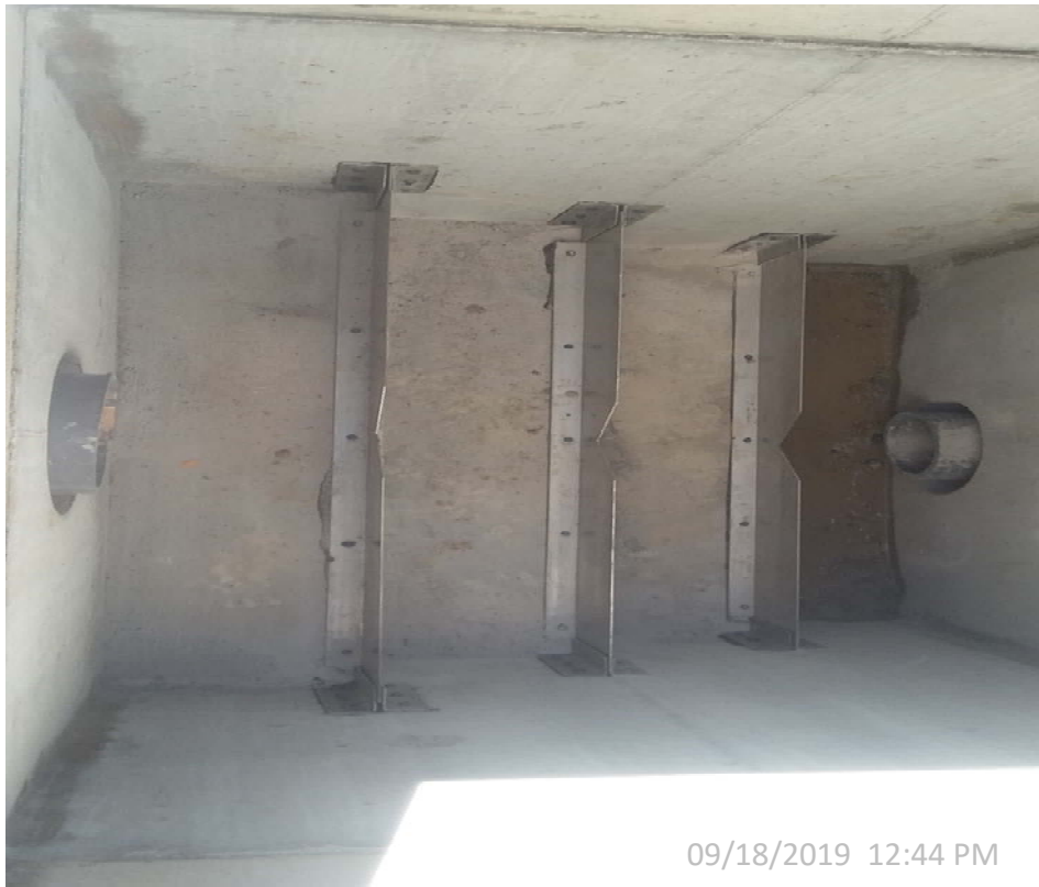
Photo 62- Settling Pond Cascade Aerator V-Notch Weirs
